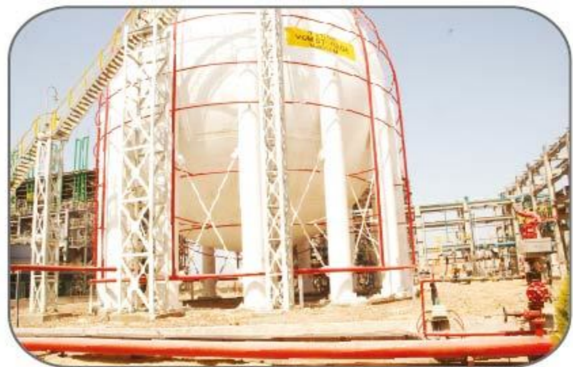
Manual and automatic operation of a cooling System for VCM-Pressurized gas spheres..
