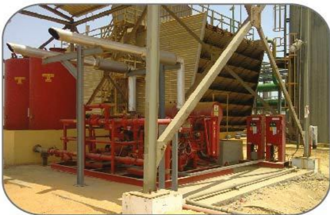
2x Foam Pump Stations ,one with 2 x electric foam pumps skid unit and 2 x diesel foam pumps skid unit , each with 20 m3 - 3%AR-AFFF foam concentrate in two atmospheric tanks.
