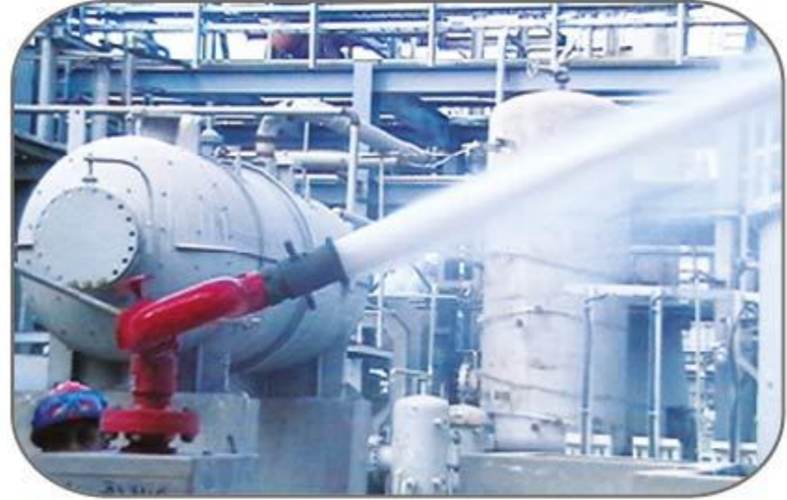
Water & Foam Monitors around the whole Factory.
